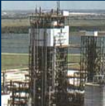
Polk County, Gasification Power Plant
